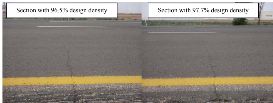
Figure 43. Observed Reflective Cracking of RAS Test Pavements on US87, Amarillo.
