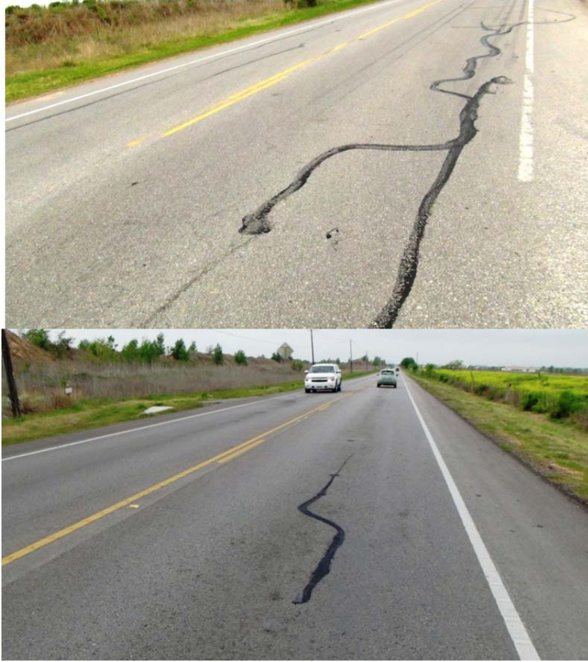
Figure 54. Cracking Observed on FM973.
