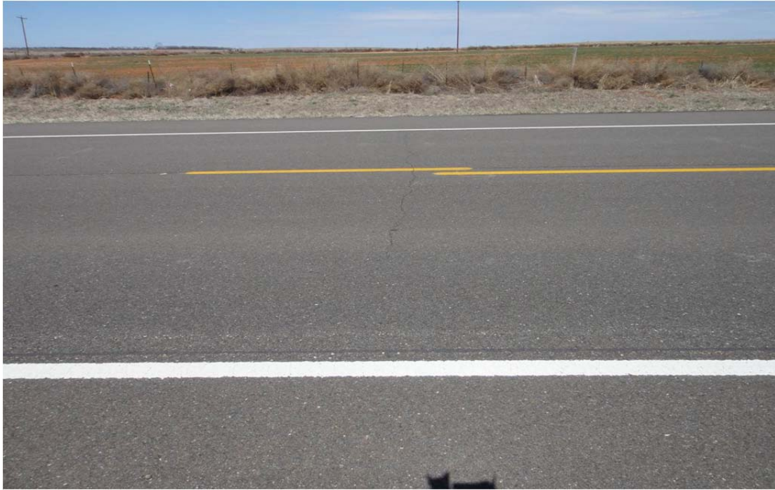
(3) Section 3: RAP/RAS Mix with PG70-28-Transverse Cracking.
