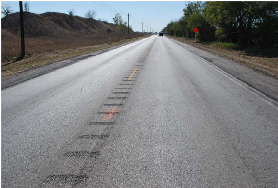
Figure 52. Typical Distresses prior to Paving at Test Section.
