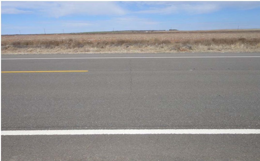
(b) Section 2: Virgin Mix with PG70-28 - Transverse Cracking.
